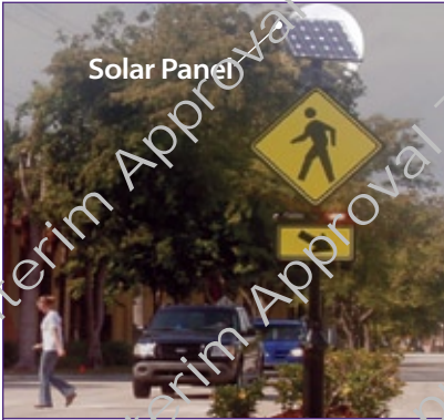
Figure 1: Activated, solar-powered RRFB on a center island at an unsignalized intersection—beacons flash using an irregular flash pattern that is similar to emergency flashers on police vehicles
